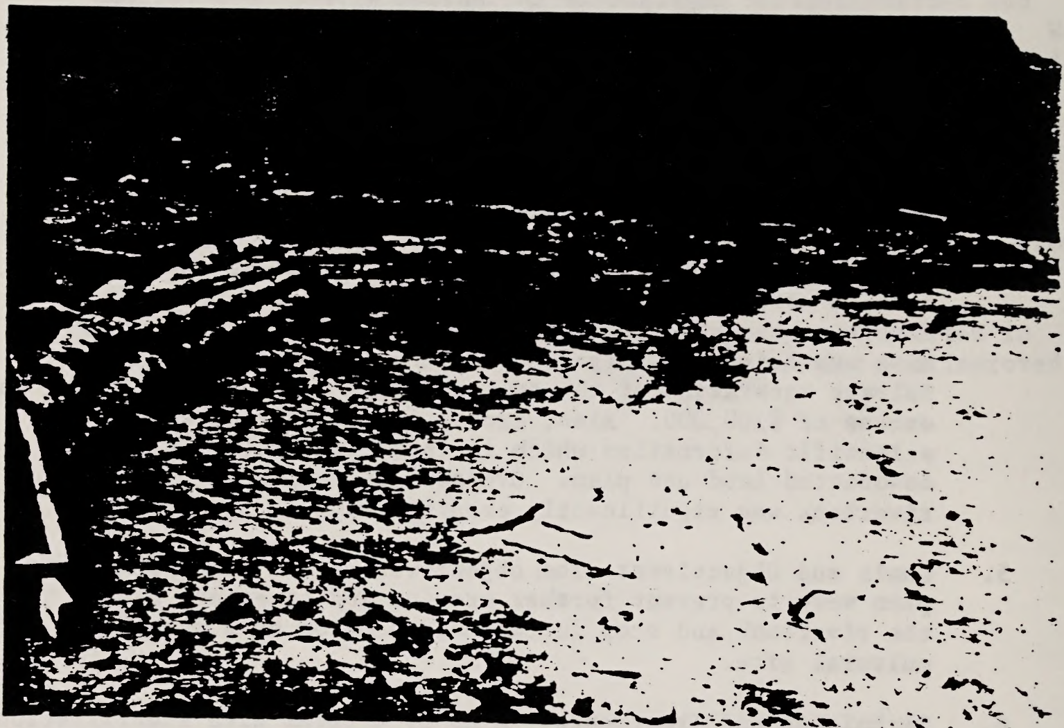
During the spring of 1985, log revetment, livestock enclosure, and seeding were used to stabilize an eroding bank along the Salmon River to protect a cultural site. High spring river flows were eroding the riverbank.
